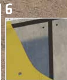
Leaking Compartment Membrane System
