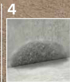
Leaking Areas of Voids i.e. Honeycombing
