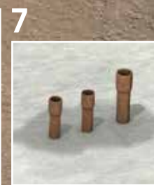
Leaking Penetrations i.e. Pipe Penetrations
